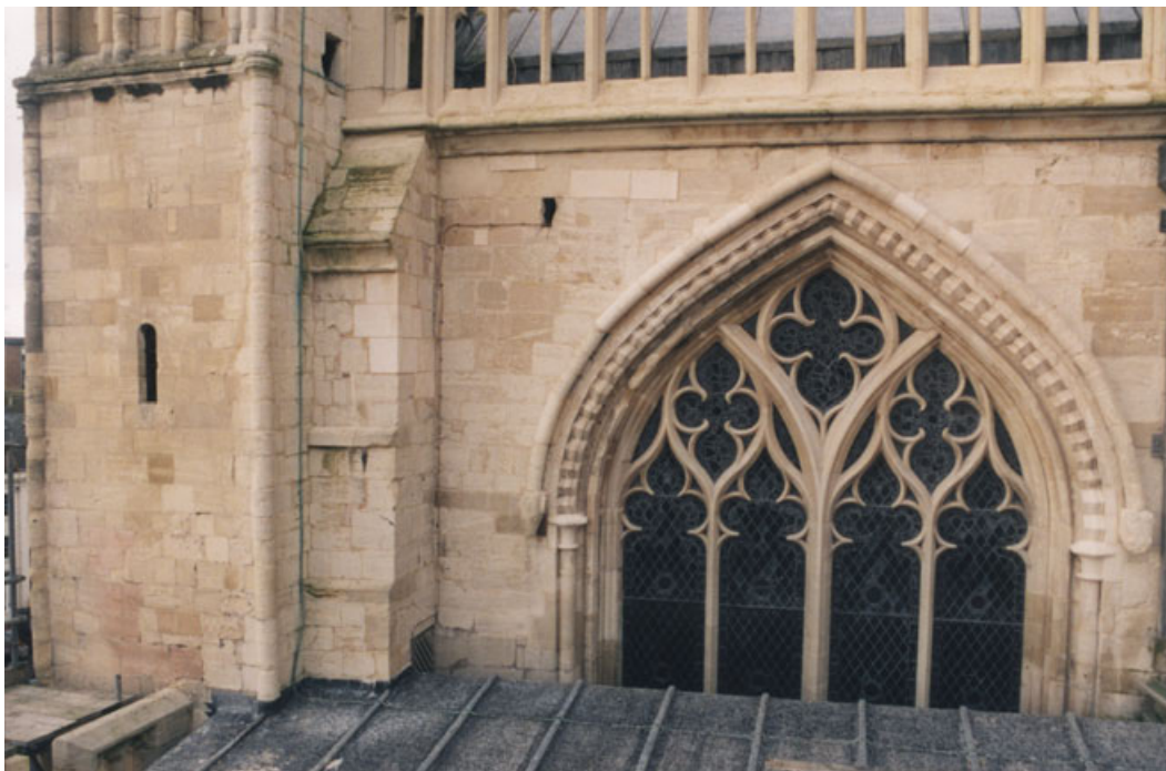
Plate 1 East side of south transept in 1999, after repairs. The remains of the Romanesque passage at clerestory level can be seen at the base of the buttress. Photo: Alan Norton.
