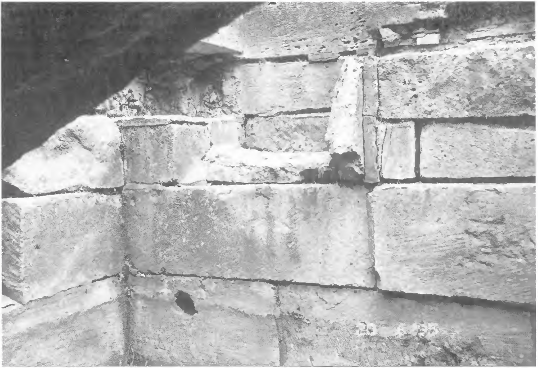
Fig. 8. View of the tank's east wall showing the culvert entrance and the hole in the lowest course.
