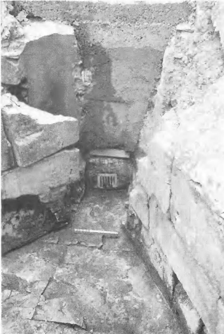
Fig. 6. View to west of the sluice with the Victorian grille beyond; the concrete manhole above the grille was the repair of 1996. The Victorian 'shaft' is left of the grille.
