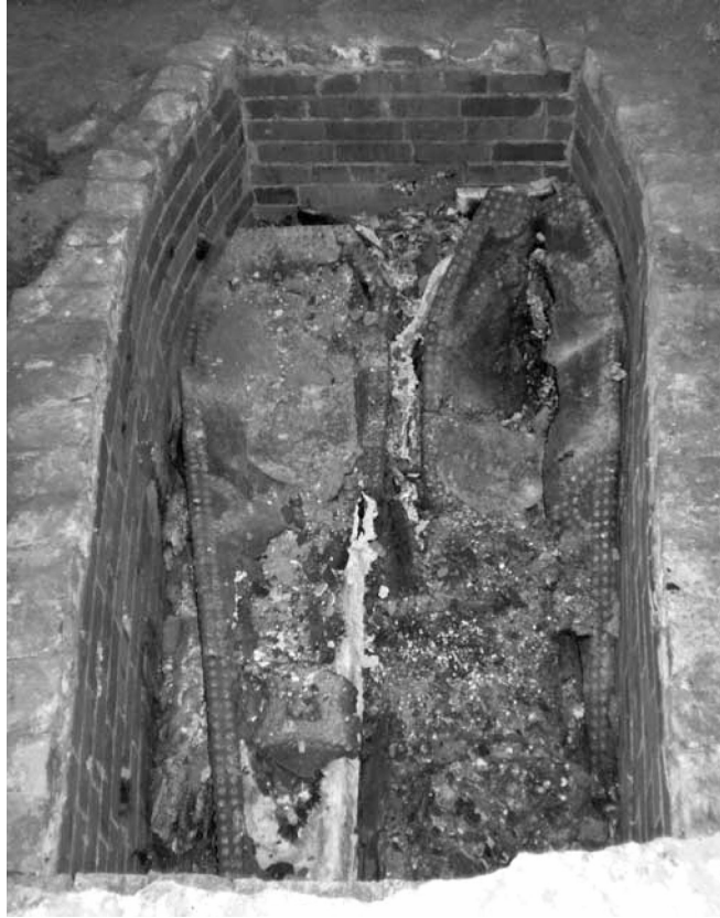
Fig. 11. The double Clutterbuck and Cripps vault after removal of the cover slabs.
