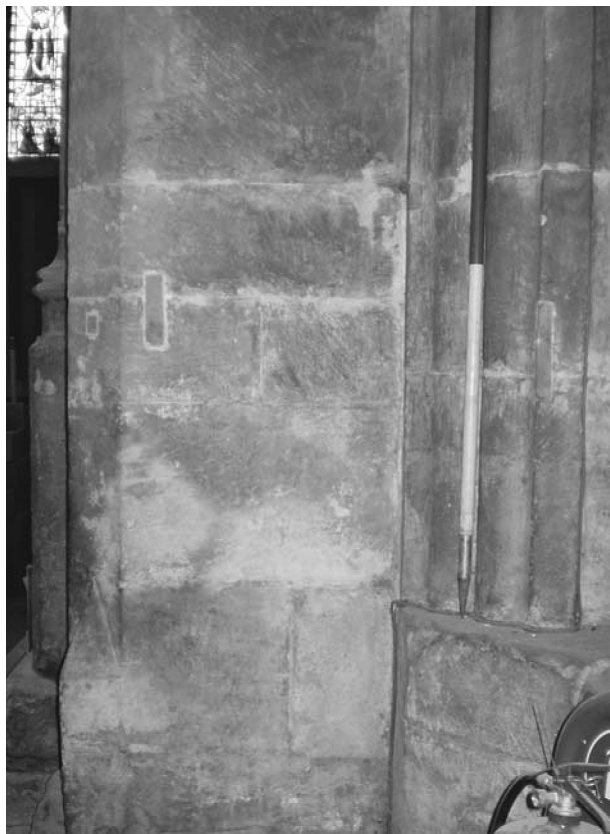
Fig. 7. The base of the southern tower arch jamb, showing junction of early and later work (to left and right, respectively), and broach stop to chamfer.
