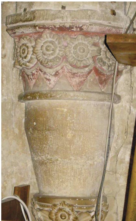
Fig. 6. The Romanesque capital and cut-back shaft of the western respond of the south chancel arcade.
